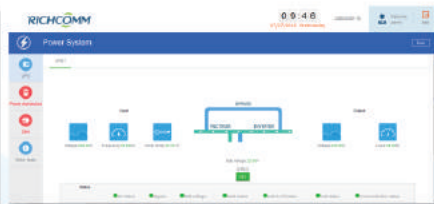
Single-phase UPS Monitoring
